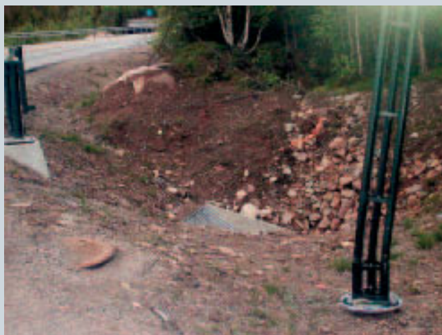
RV 23 the Oslofjord Connection. Road equipment is placed where the probability of running off the road is greatest, at the exit from the roundabout.
