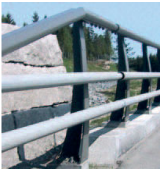
Guardrail with sharp edges and inferior curb termination
