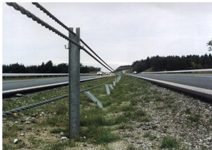
Wire Rope Safety Fence: here, one of the cables is not in place, following an accident
