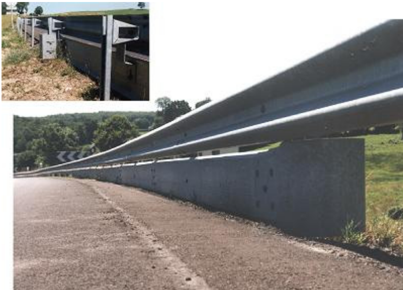
On a French road, a second lower flat rail is fitted under the armco (above: rail seen from behind)
